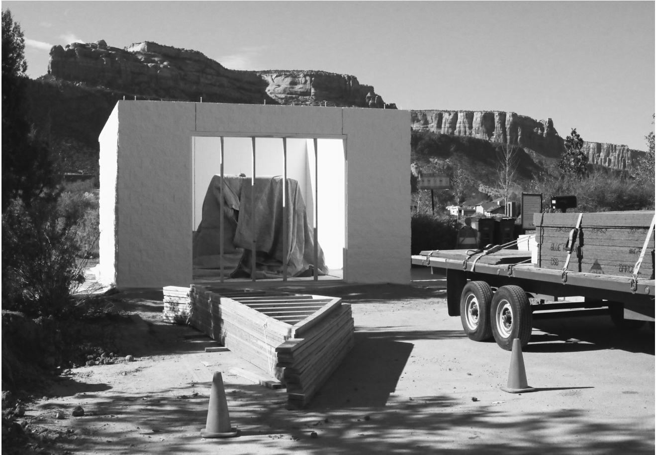
Above Photo by John Eklund - Pump station building under construction as part of the Monument Valley Pump Station Improvement Project in the Redlands area.
